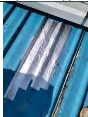
Penambalan korosi atapselasar ged. terminal
