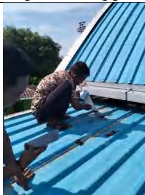
Penambalan korosi atapselasar ged. terminal
